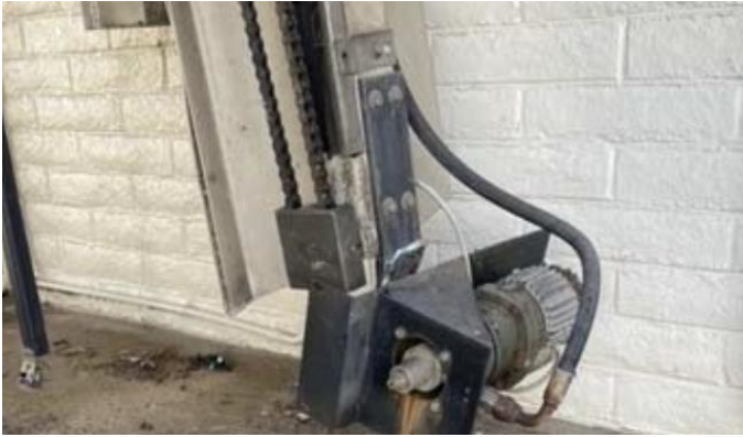
Evidence of vehicle impacting the Gantry.
