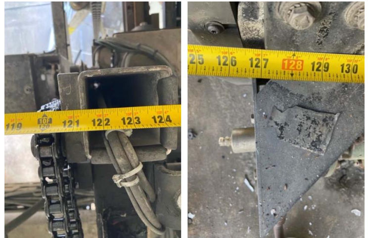
Due to the impact, the Gantry Frame Assembly has been stressed beyond its design. The Gantry Frame Assembly has been bent several inches from the top of the structure to the bottom as pictured above.
