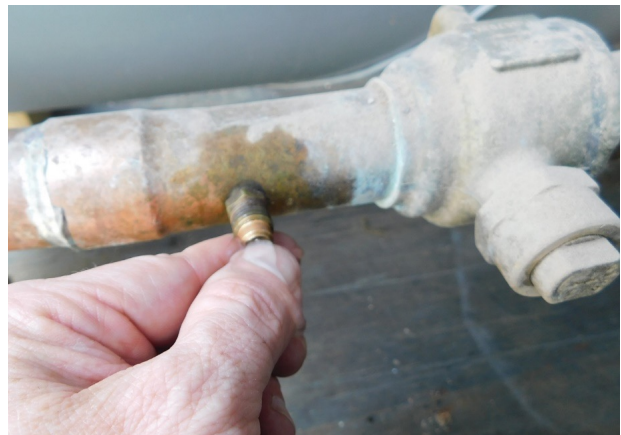
Water coming out of the refrigerant line valve for the chiller.
