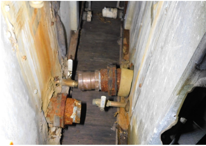
Corrosion to the air handling coil connections, which is not a result of the water line failure.
